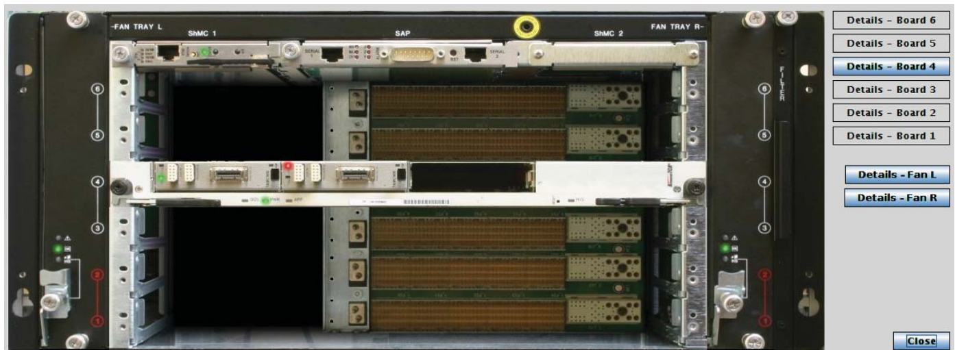
Fig. 3. A graphical software representation of the shelf front panel. The monitored shelf contains two cooling units and a Carrier Board with two AMCs.
